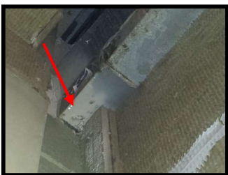
Water leaking into stockroom below
